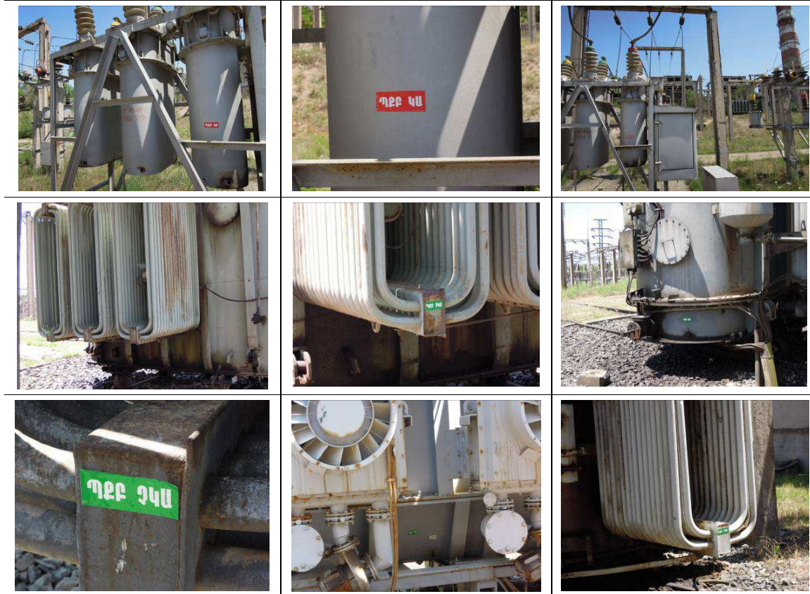
Facility: TEC Yerevan – electric power plants, old facility
